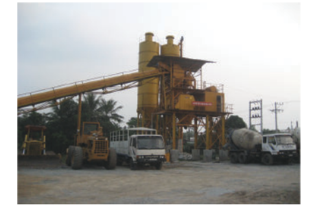
Ready-mix concrete mixing plant
